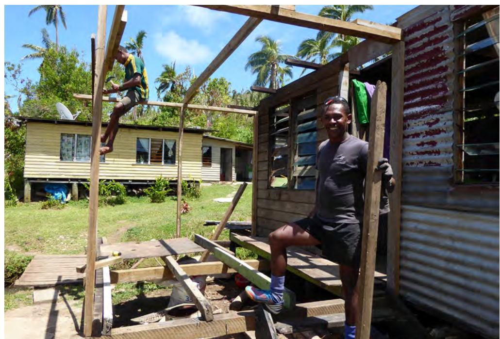
Neighbours help rebuild each others' houses after Tropical Cyclone Winston hit Nukubalavu village in Savusavu District, Fiji, in March 2016. The Category 5 Cyclone was the biggest to ever hit Fiji and killed 44 people. © Holly Griffin/IFRC
