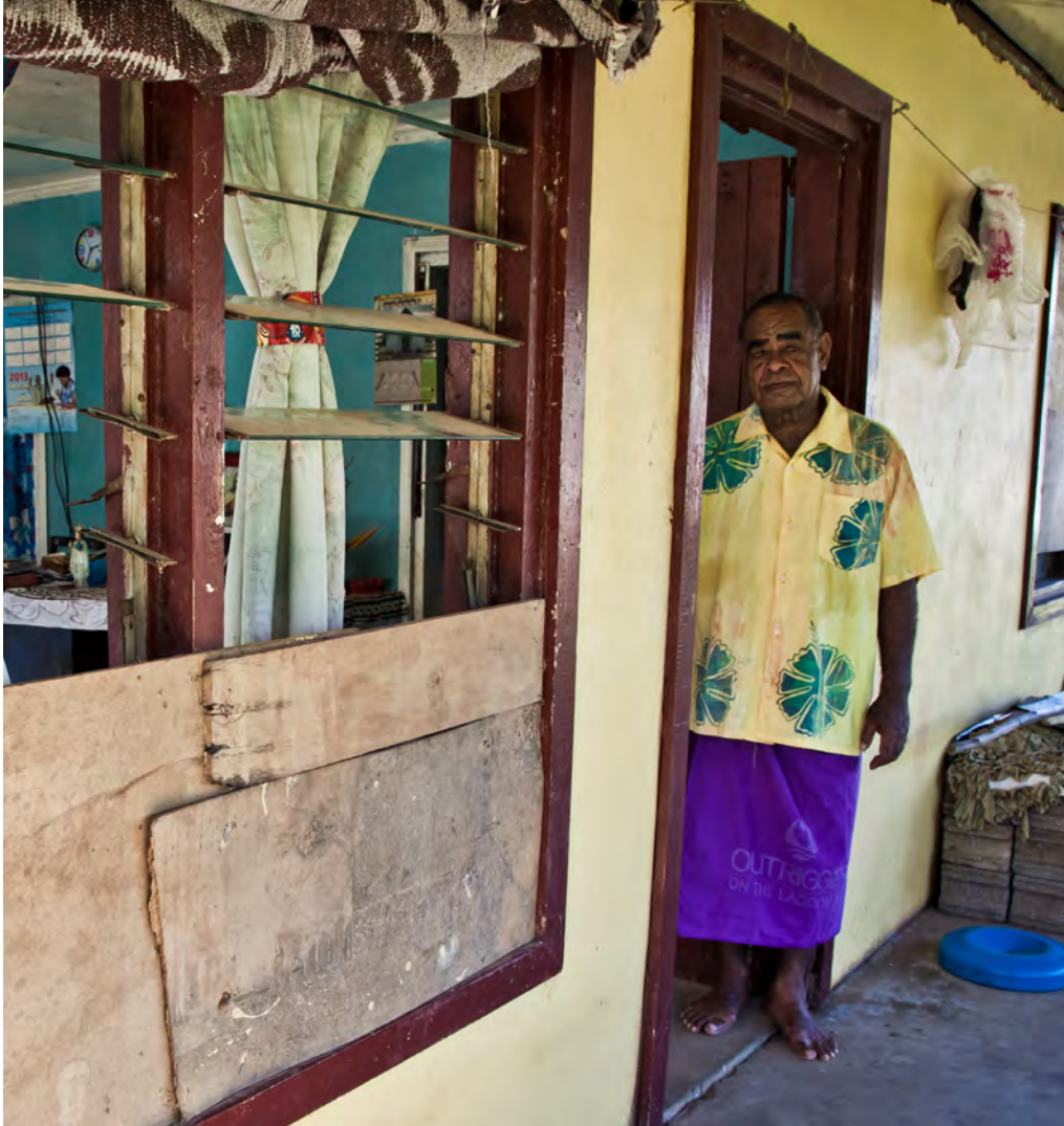
A local man stands in his home located near a river in Votua Village, Ba town, Fiji. His home is frequently flooded as the level of the river has been increasing every year due to erosion of the surrounding mountains. © Benoit Matsha-Carpentier / IFRC
