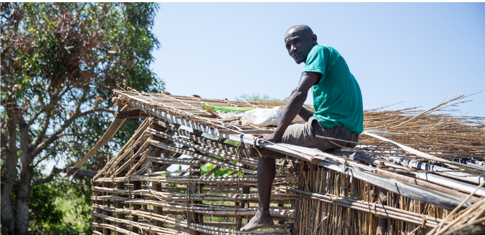
Photo 3: Local resident rebuilds his damaged house in Nhagueira, Sofala province. Source: IOM Mozambique
